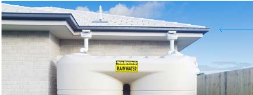
Rainwater capturing techniques: rainwater catchment system
