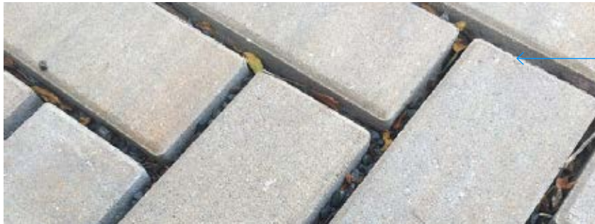
Rainwater capturing techniques: permeable pavement
