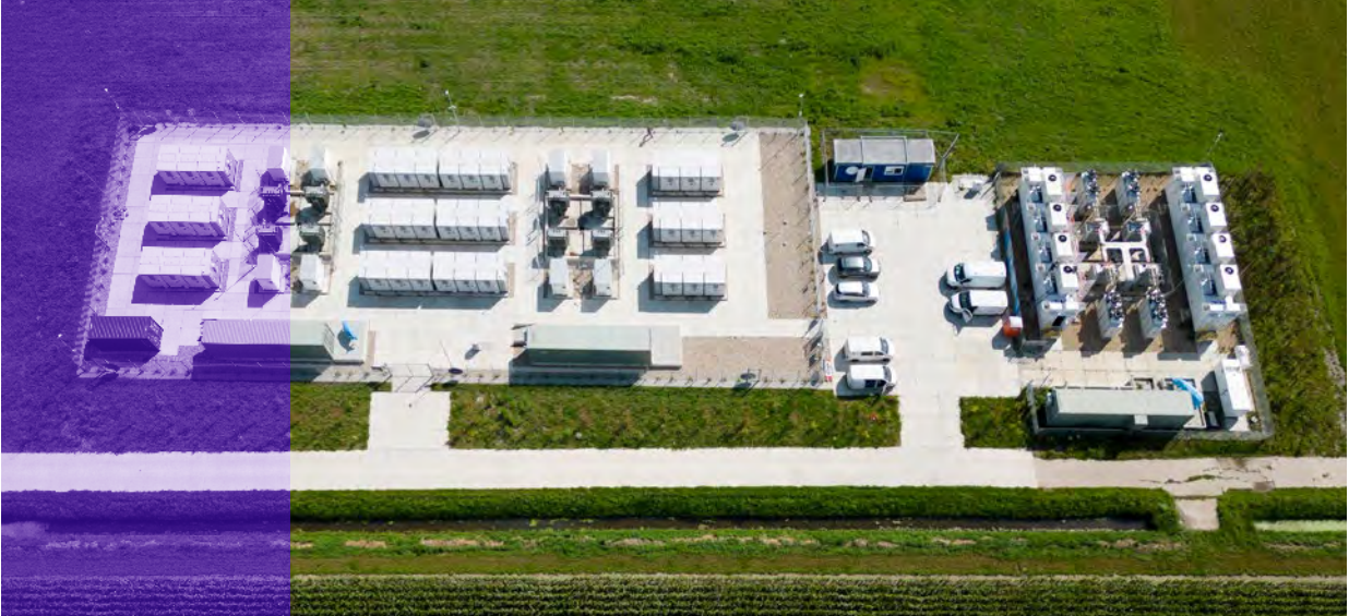
Chemical battery facility Flevopolder, The Netherlands
