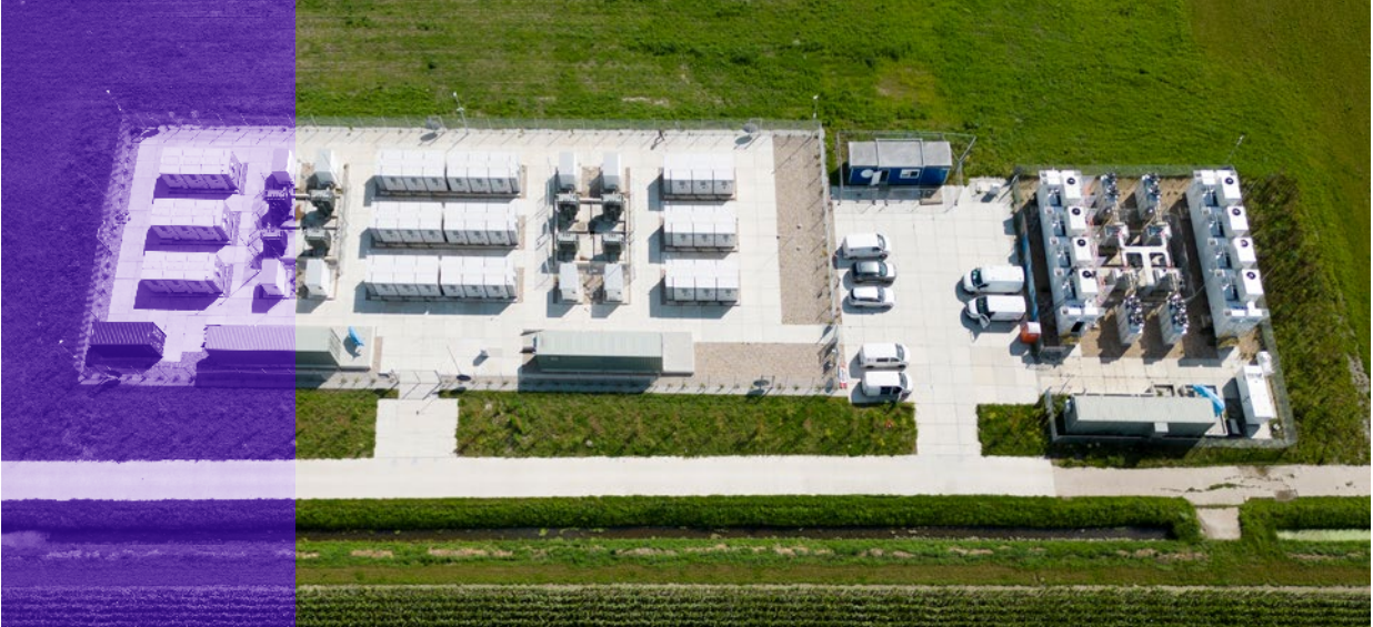
Chemical battery facility Flevopolder, The Netherlands
